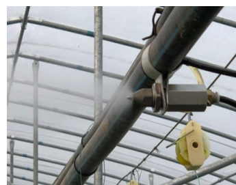
c. Twin-fluid nozzle in greenhouse
