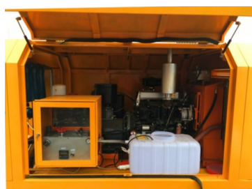
a. Control unit of spraying system
